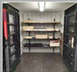
Storage for spare parts
